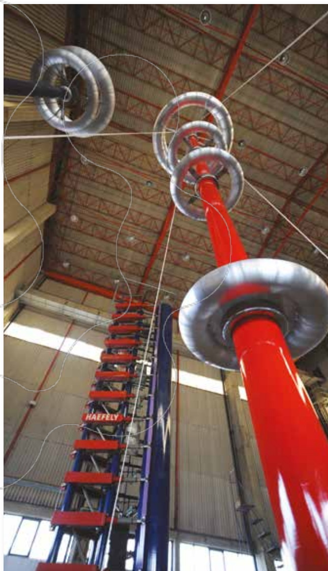
Lightning impulse generator voltage divider.
