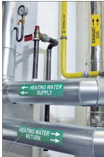
Large and highly visible pipe marking.
